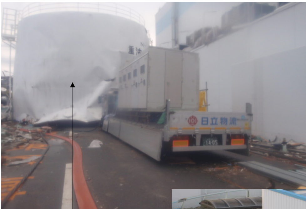
A heavy fuel tank has been drifted, and has completely blocked the road.
