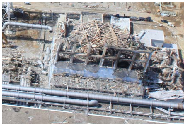
Reactor No. 3 (East side) Hydrogen built up in the 5 th & partially in the 4 th floor (north-east)
